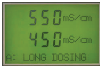
Long-dose alarm warns of dosing systems faults
